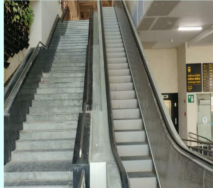
Escalator at Station Entrance
