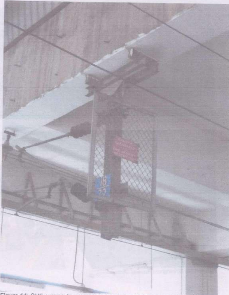
Figure 14: OHE suspension arrangement at DMRC's Tughlakabad station (1)
