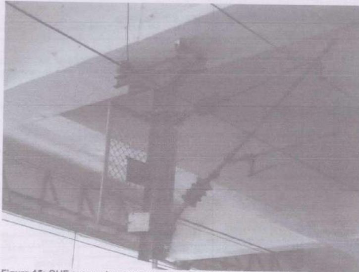
Figure 15: OHE suspension arrangement at DMRC's Tuglakabad station (2)
