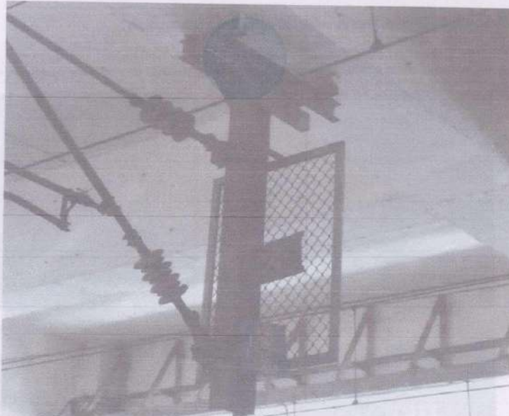
Figure 16: OHE suspension arrangement at DMRC's Tuglakabad station (3)
